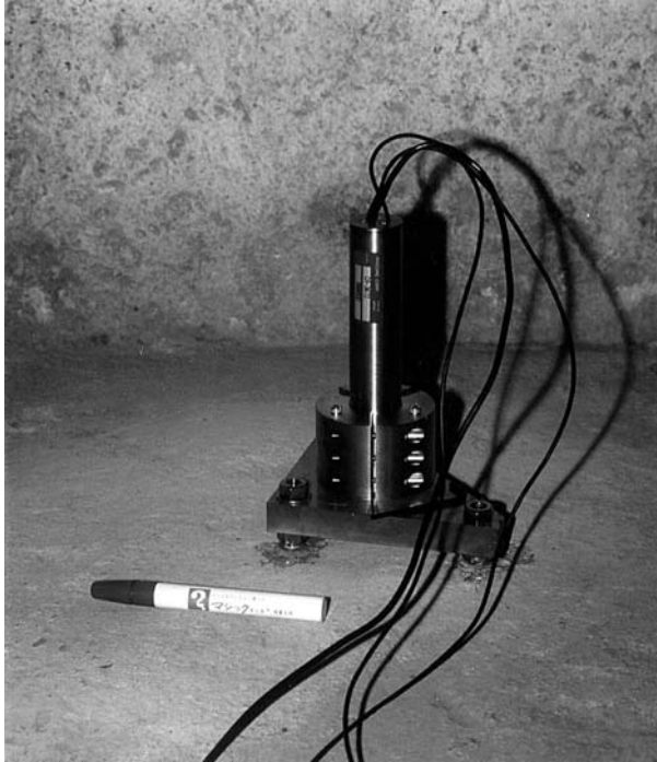
Fig. 2 The picture of the tiltmeter (CA-3672) installed on the floor.
